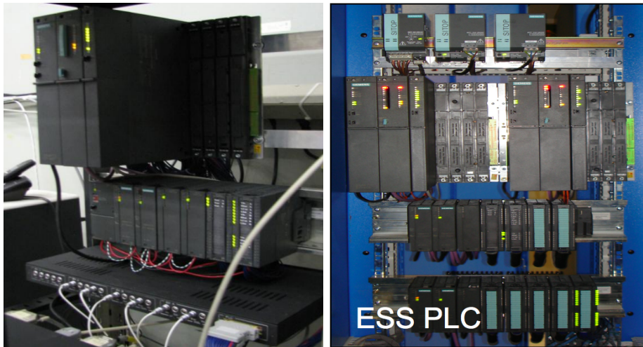
Figure 4.6: A photograph of the ESS PLC system and an interlock unit configured as described in the text, installed in the ECAL Integration Centre (left), and a photo of the ESS PLC system in stalled at the UXC area at P5 (right).
